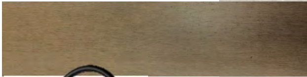
Cabinet Stain @ Perimeter
